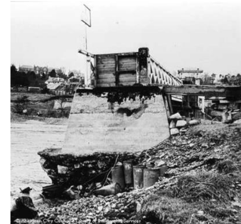
Southern end of bridge after flooding. Courtesy Aberdeen City Council - Silver Vault
